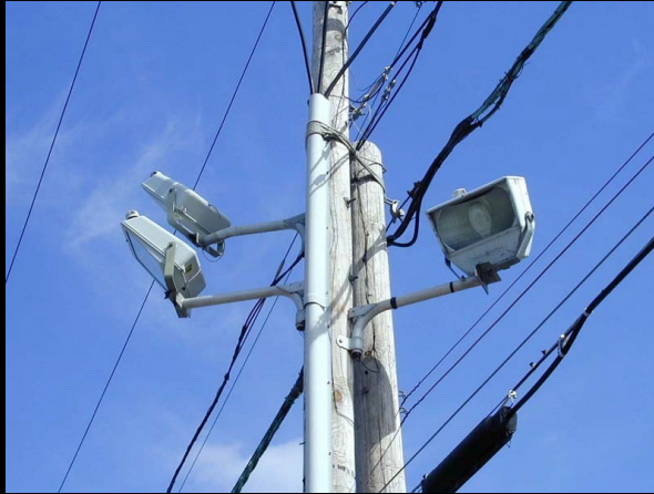
Pole-mounted 400-W floods
