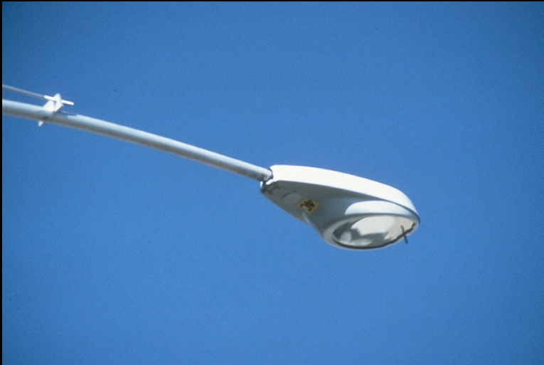
Fully shielded road light
