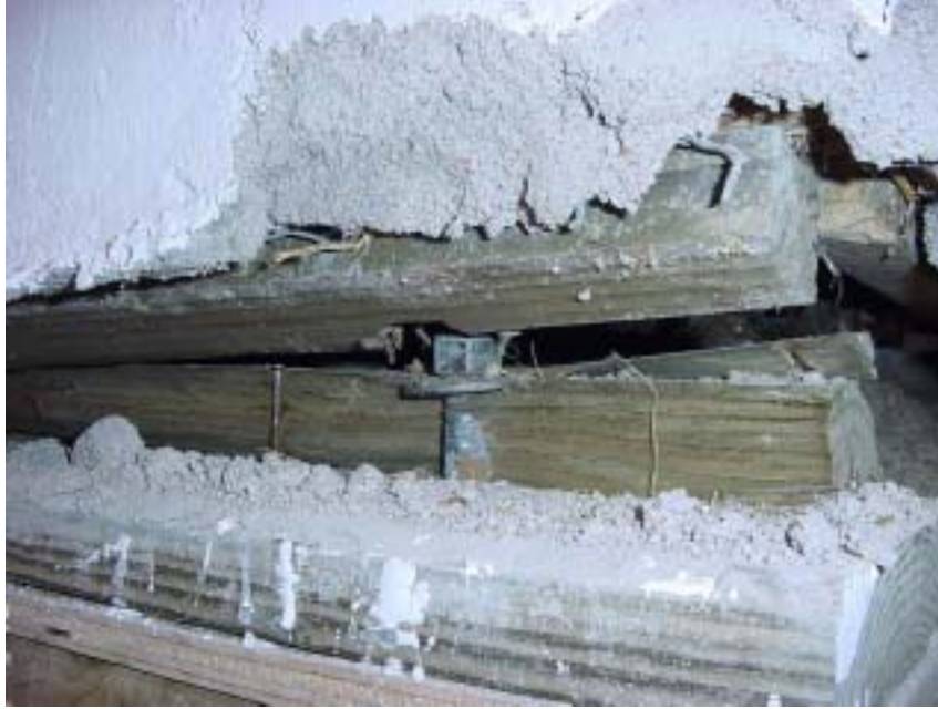
Figure 6.6 – Wall D cross-grain bending failure of sill plate (Photographed at 5% drift, well after failure had occurred)
