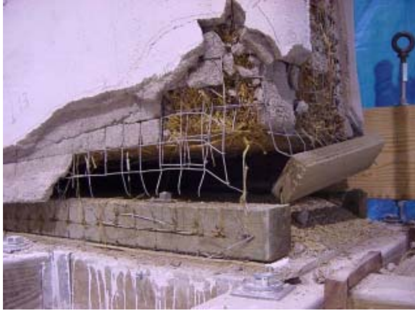
Figure 6.9 – Wall E mesh failure (7.5% drift level)
